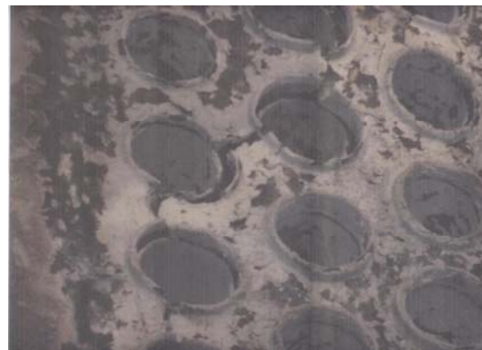
Fig.6 View of a part of the damaged tubesheet
