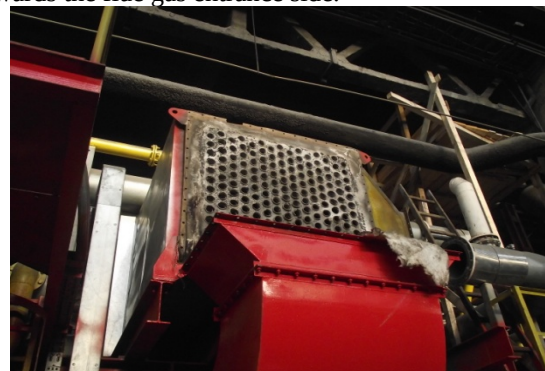
Fig.5 View of the air pre-heater, from the flue gas entrance side towards the damaged tubesheet
